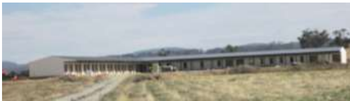
One completed wing of the new convent in Tynong blessed before Lent by Fr. Fullerton, the Australian District Superior
